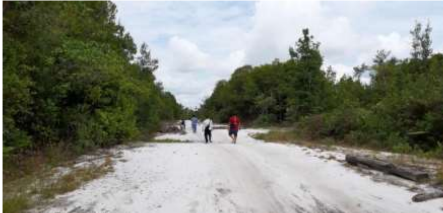
Figure 2. Condition of the Danau Rawah Village - Timpah Road Section, Kapuas District
